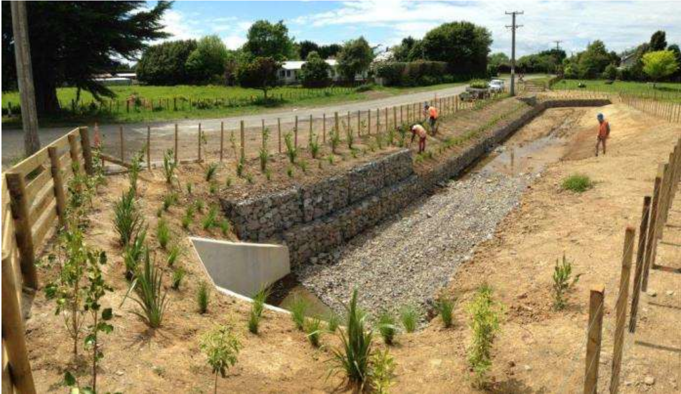
Planting and reinstatement around the outlet (November 2017). TMP – temporary traffic light in operation (November 2017)
