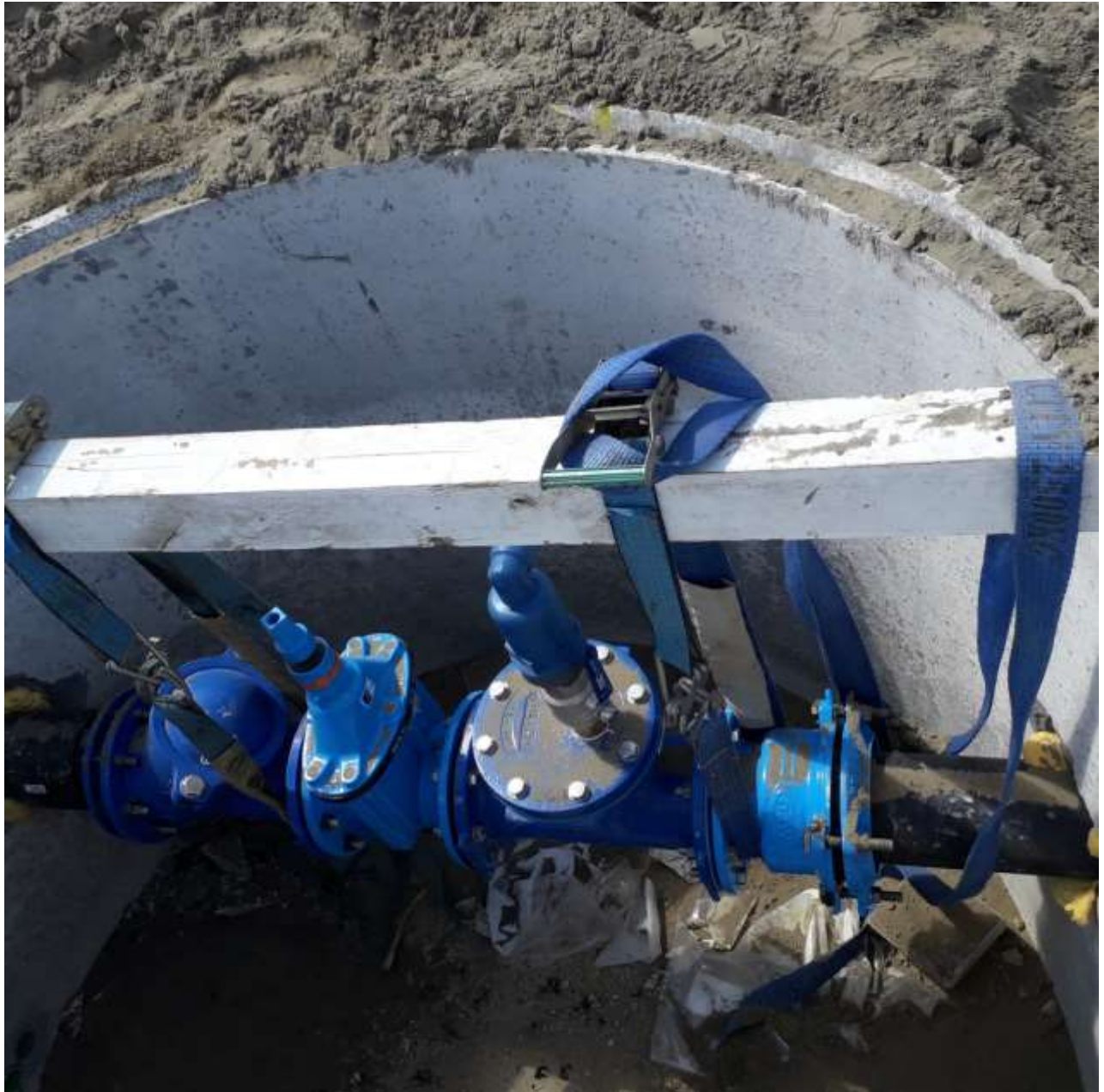
Okarito pumpstation valve chamber (November 2017).
