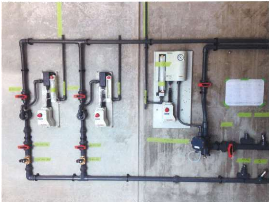
New chlorine dosing equipment (Feb 2017)
