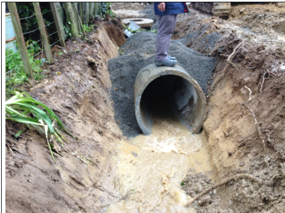
New 750 mm pipe being installed to connect water race to new pipeline.
