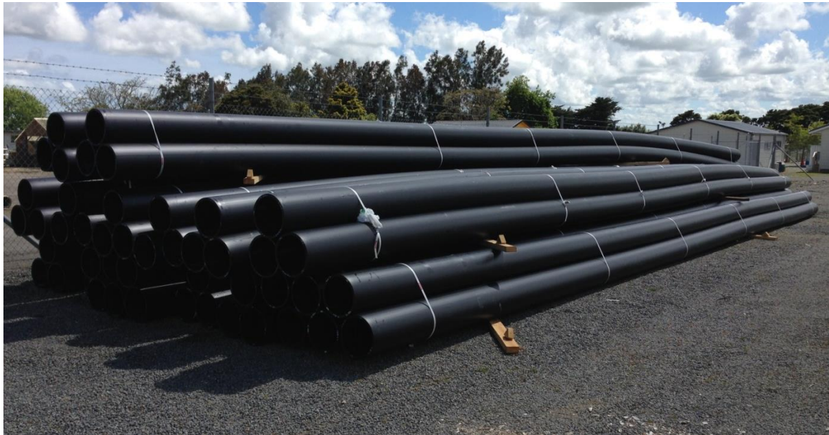
Kennedy Drive rising main pipes delivered to Downer yard (Hokio Beach Road – October 2016).
