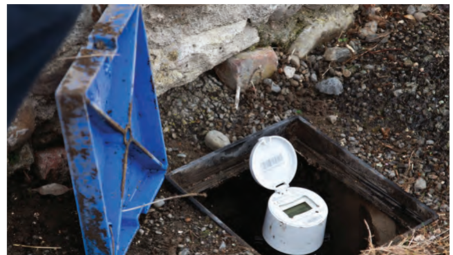
Distinctive blue-topped water meter
