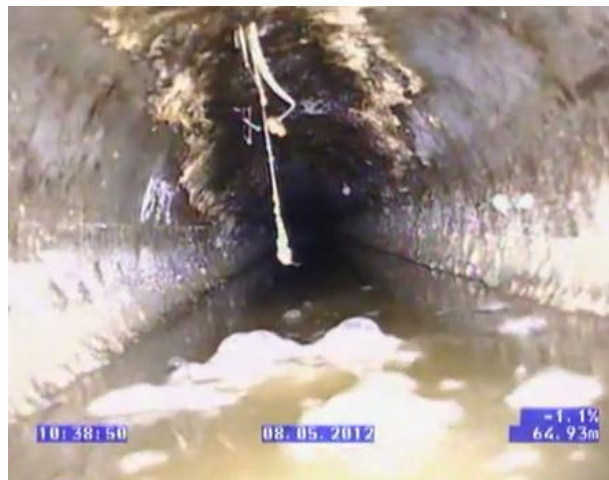
What lies beneath us - a blocked and broken wastewater main under Stafford Street, Shannon 2012
