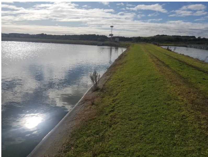
East bund of the second pond in 2019. The wavebands are visible above the waterline and the bund above the waveband is in good condition.
