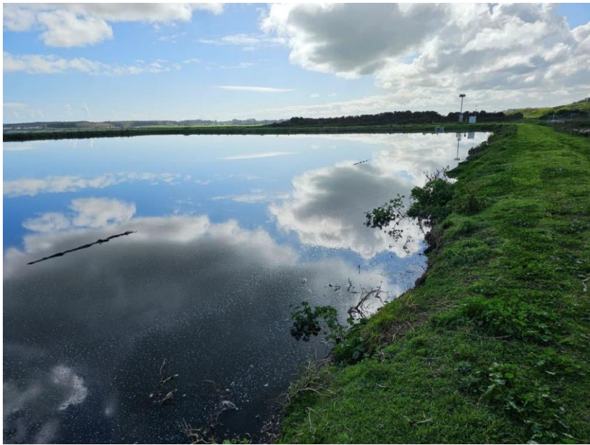
East bund of the second pond in 2024. The wavebands are submerged, and the bund shows the signs of wave erosion and loss of formation.
